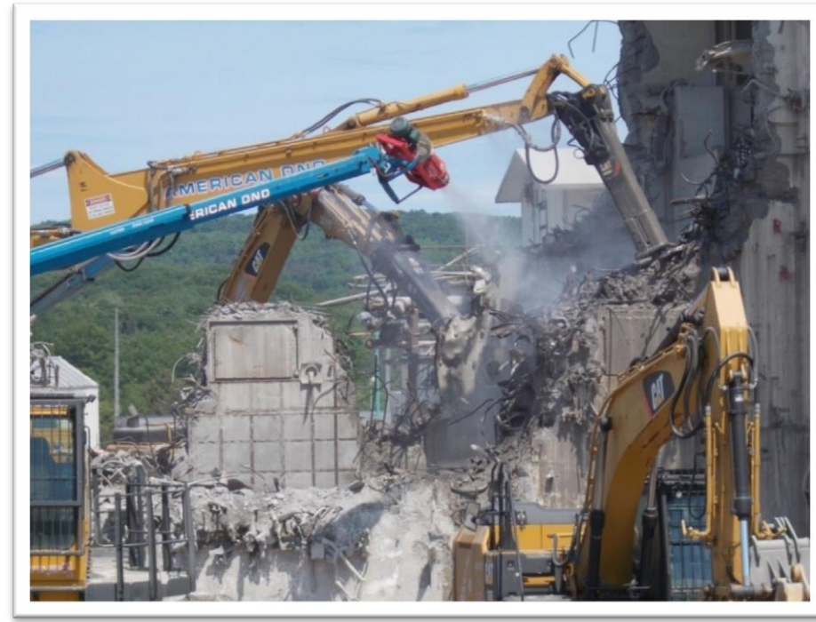
Vitrification Facility Demolition Excavators with hydraulic hammers demolish west and east walls
